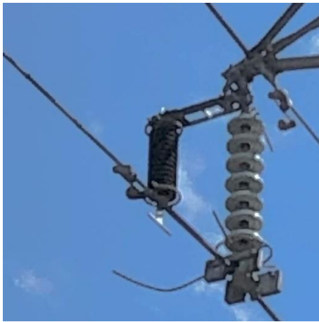
(a) Metal-oxide surge arrester
