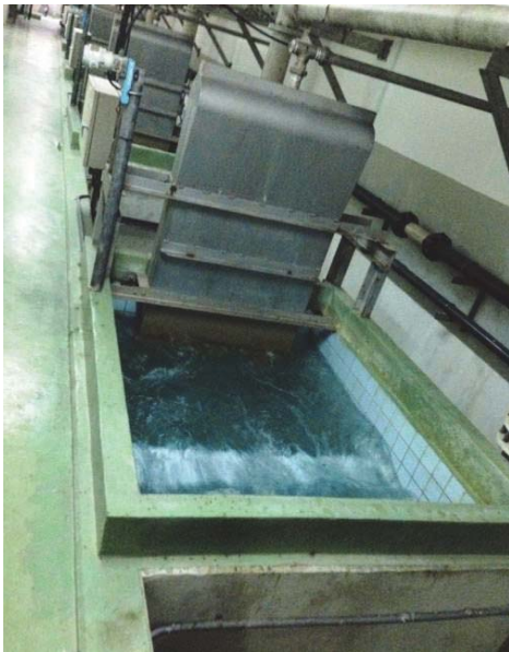
Fig. 7 Chlorine dosing basin
