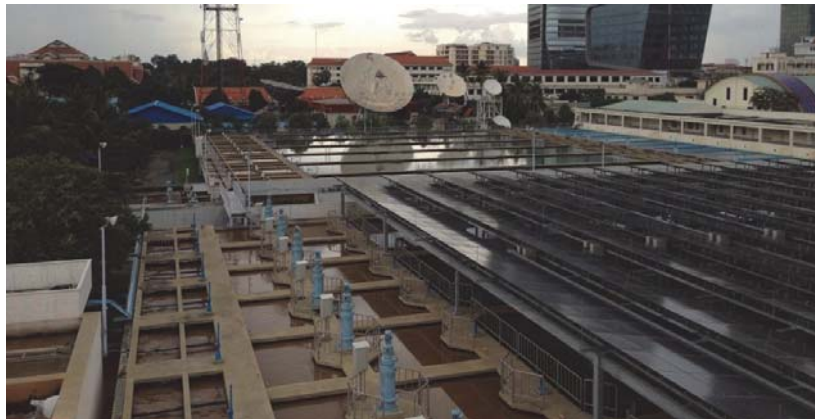
Fig. 2 Phum Prek Water Treatment Plant
