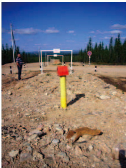
Photo 1 A view of the ESPO pipeline-buried route in the midst of taiga forest at the suburb of Neryungri city, Sakha Republic (August, 2010).
