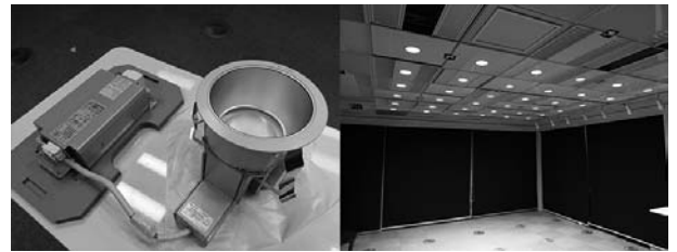
Fig. 3. Cut-off downlight with narrow luminous intensity distribution of 49° (left). The experiment room in which the cut-off downlights are installed at interval of 0.6 m (right).
